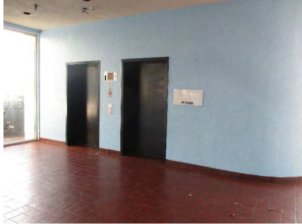
Photograph 18. View of the two elevators within the on-site building. Elevator pits were inaccessible.
