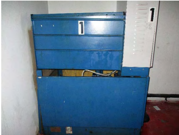
Photograph 19. View of the elevator room located on the first floor. Photo shows typical hydraulic unit for elevators.
