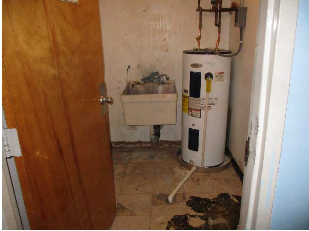
Photograph 21. View of the typical utility room and floor drain. Photo shows the first floor utility room and associated stain.
