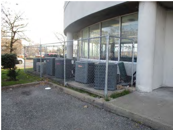
Photograph 11. View of the HVAC system located within a fenced area in the northwestern portion of the subject Site.
