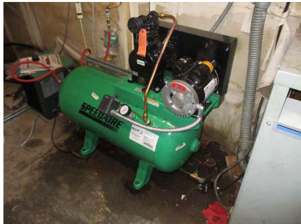
Photograph 16. View of the 80-gallon electrical air compressor horizontal tank located within the electrical room.
