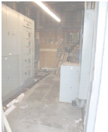
Photograph 15. View of the main electrical room for the subject Site building. Photo taken from doorway.
