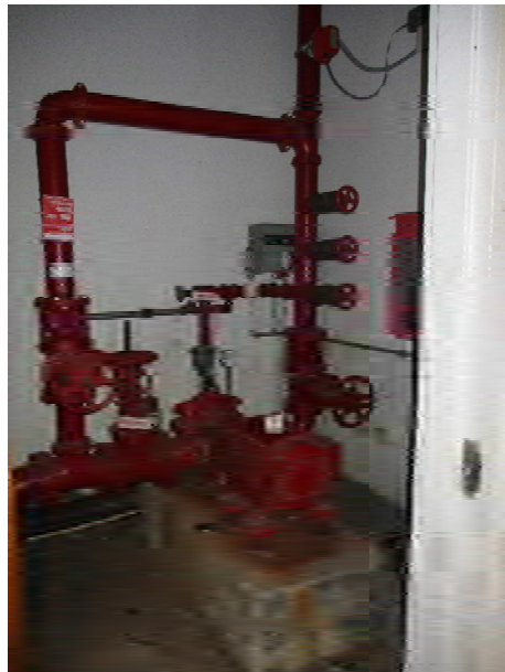
Photograph 20. View of the sprinkler room located on the first floor.
