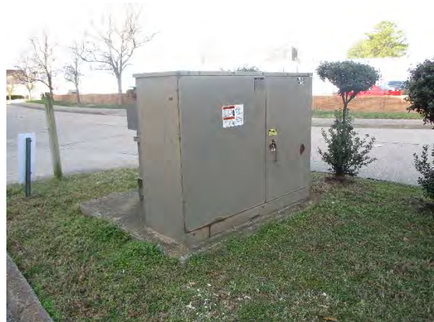
Photograph 12. View of non-PCB electrical transformer located in the northwestern portion of the subject Site.
