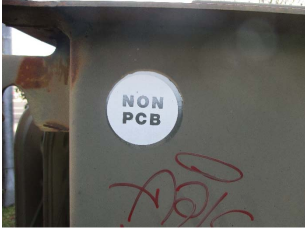
Photograph 13. View of the Non PCB placard affixed to the electrical transformer.
